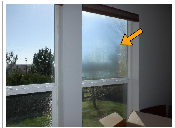
Figure 10.4 - Fogging or staining between glass panes at dining area.
