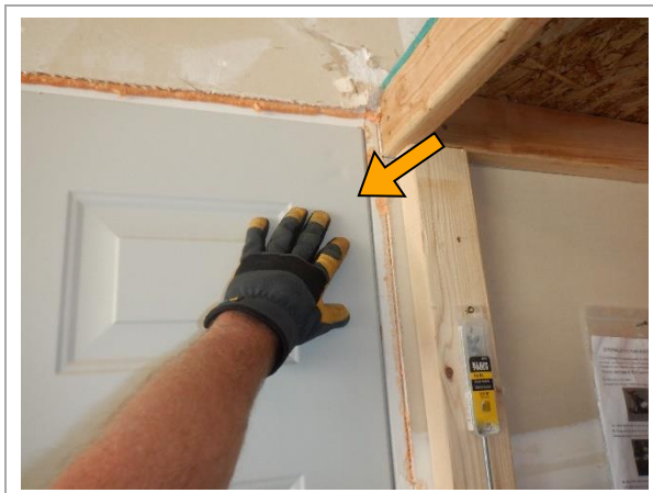
Figure 10.5 - East garage door drags against its frame.
