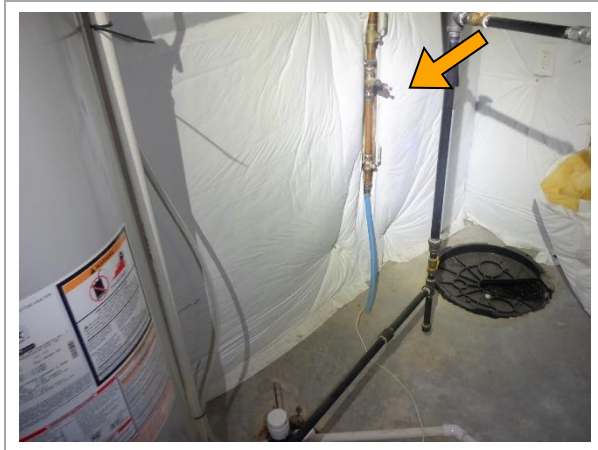
Figure 6.1 – Main water shutoff valve in basement mechanical area
