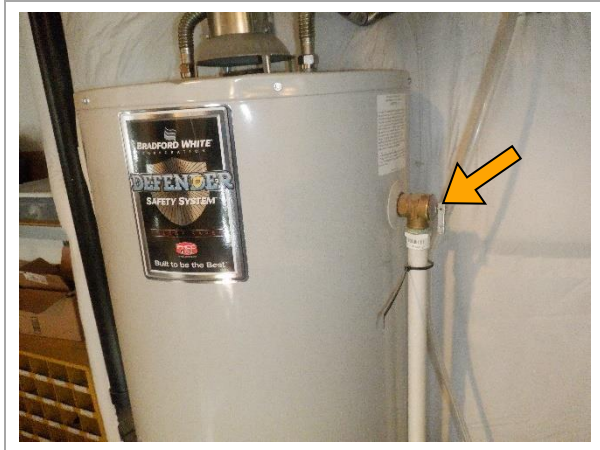
Figure 6.7 – Pressure/temperature relief valve verified at water heater
