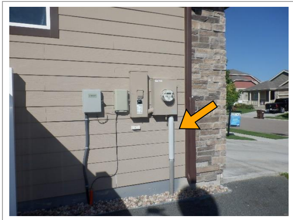
Figure 7.1 - Electrical service entrance at south exterior
