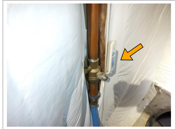
Figure 6.2 – Main water shutoff valve (2 nd view)
