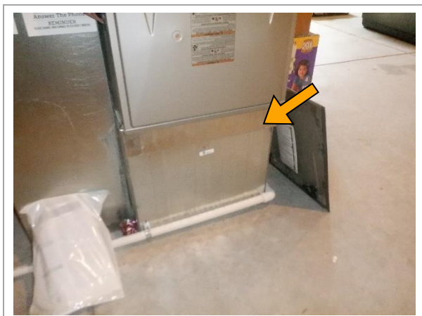
Figure 4.5 – Furnace/HVAC filter access
