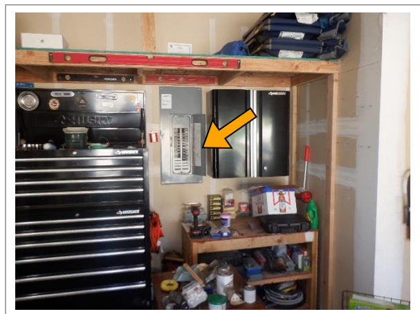
Figure 7.4 - Breaker panel location in garage area
