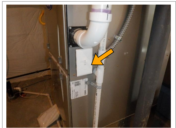
Figure 4.4 – Presence of electrical disconnect verified at furnace
