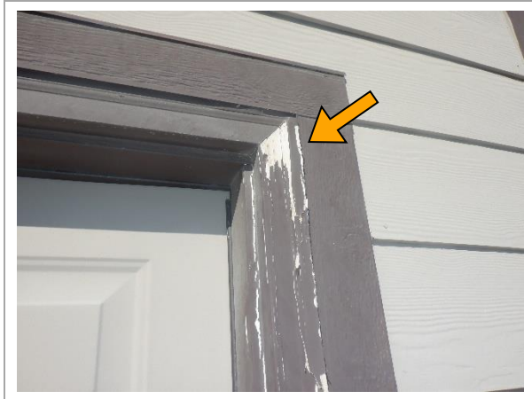
Figure 2.1 – Example paint/finish deterioration.
