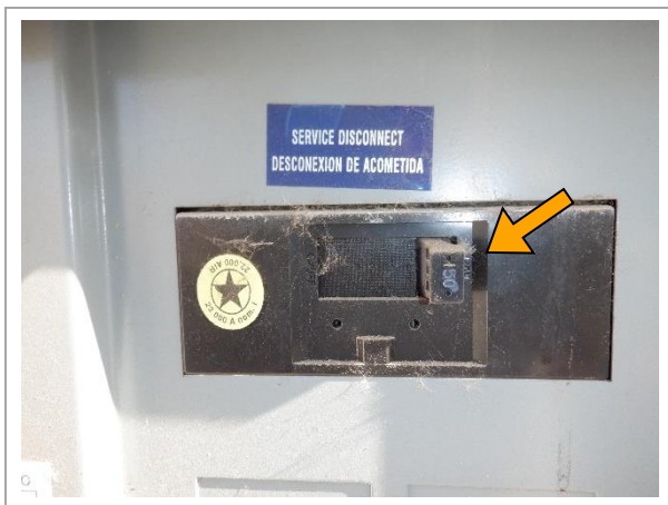
Figure 7.3 - Electrical service main disconnect (200 amp)
