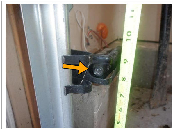
Figure 10.3 - Garage door photo sensors higher than 6 inches above the floor.
