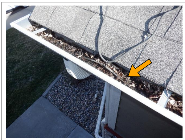
Figure 1.5 - Leaves/debris in gutter system.
