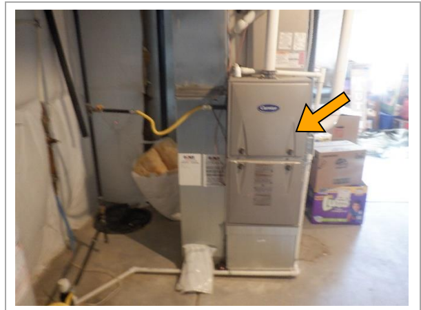
Figure 4.2 – Location of furnace in basement mechanical area
