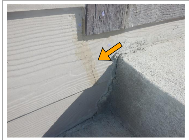
Figure 2.2 – Example cracked wall covering plank.
