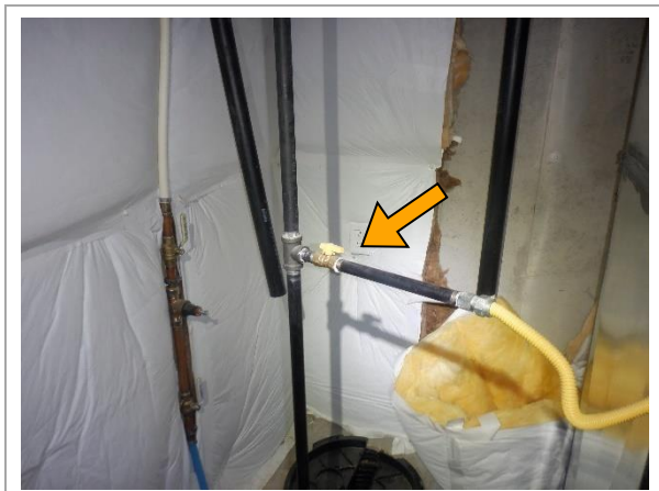
Figure 4.3 – Presence of gas shutoff valve verified at furnace
